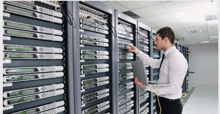
TELECOM DATA CENTER ACILIA, TIER IV 2016 Rome (Italy) Application: Data Center Plant type: Hydronic System
