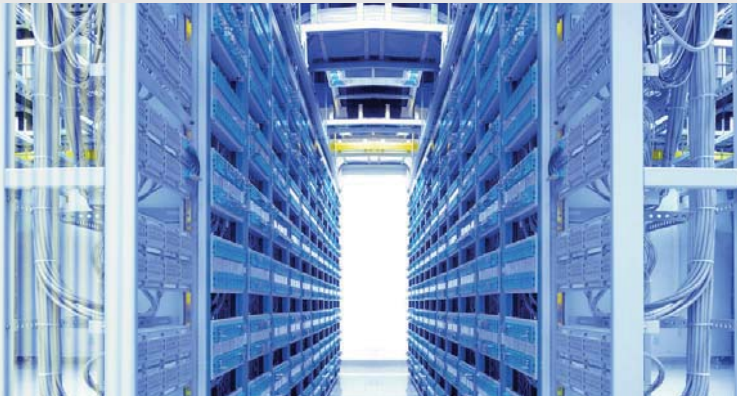
NOS DATA CENTRE 2016-2018 Carnaxide (Portugal) Application: Data Center
